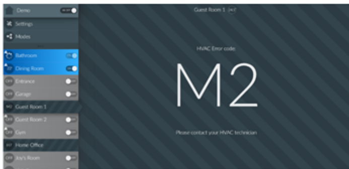
Indoor Unit Malfunctioned
